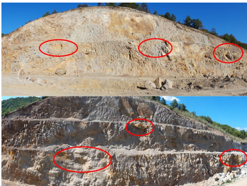
Figure 2. A look on the excavated part of the slope in the period from November 2019 (up) till September 2020 which indicates possible extension of deterioration phenomena's (down).
