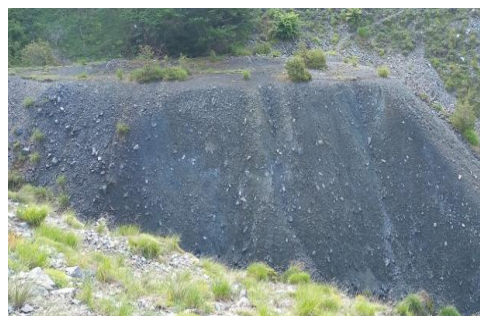
Figure 3. Remnants of asbestos-containing tailings and landfill sites in the Bajgora region are associated with historical mining activities since the 1940s
