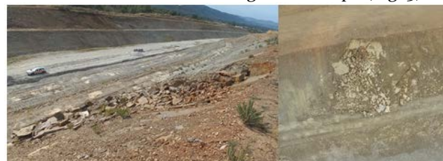
Figure 3 Rockslide state on 27.09.2023.
