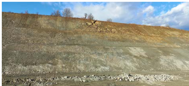
Figure 2 The initial stage of the rockslide (01.02.2023).
