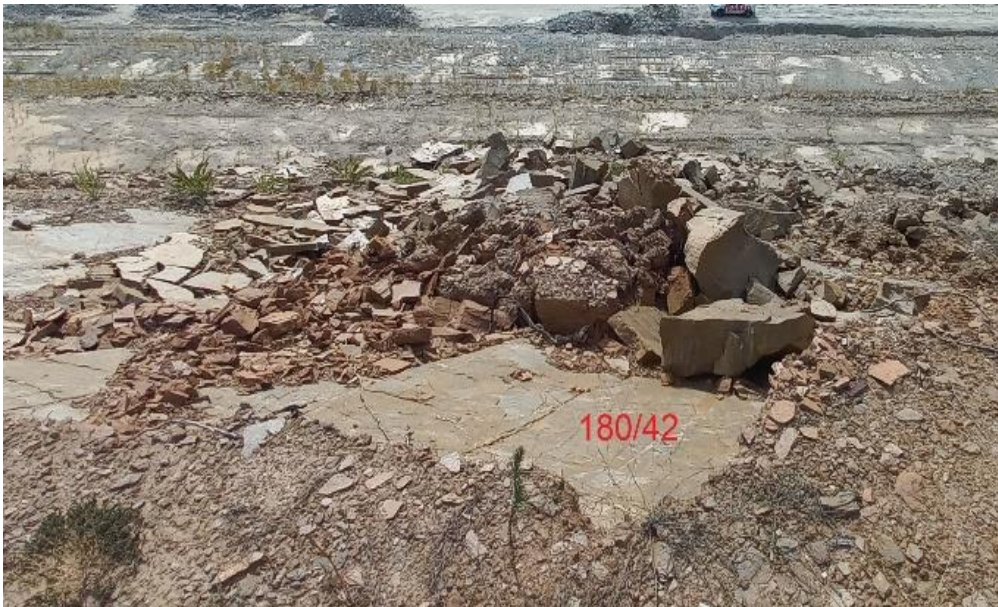
Fig. 7. The new sliding of the rocky material occurred on the upper part of the third slope with a dip direction and dip of the foliation of 180/42°
