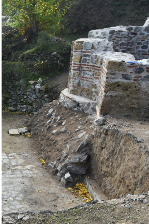
Fig. 9. Retaining wall, in front of the east wall, after closing the fugue.
