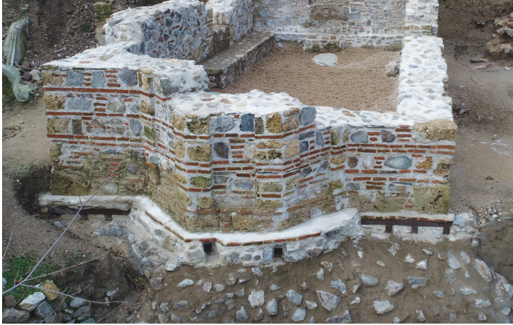
Fig. 13. East wall of the medieval church after conservation, restoration and partial reconstruction.
