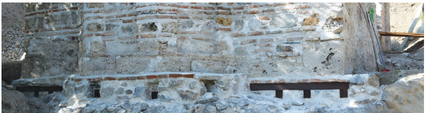
Fig. 10. Wooden beams from the Santrach system, at the east wall of the medieval church.
