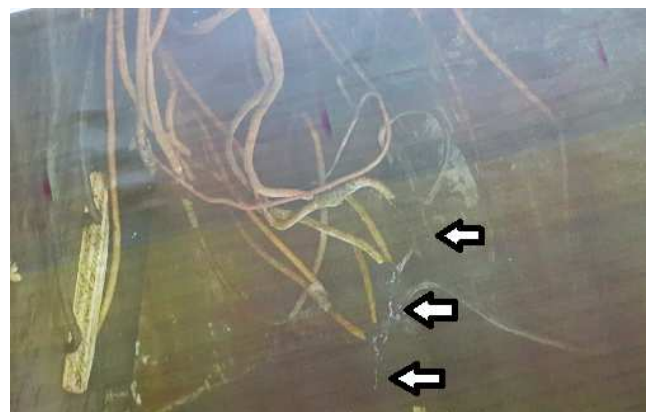
Figure 4. Connection of a meter behind a carrier board made of fiber.
