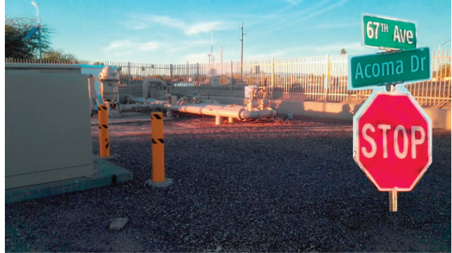
Fig. 7: Water pumping station in Glendale, AZ (photo by author)
