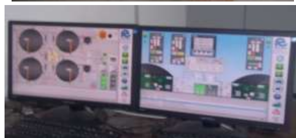
Figure 5. SCADA system (Picture taken by author 1 )
