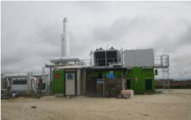
Figure 1. Part of biogas power plant in Porodin (Picture taken by author 1 )
