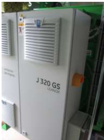
Figure 2. Genset-Container type; JGC 320 GS in Porodin (Picture taken by author 1 )
