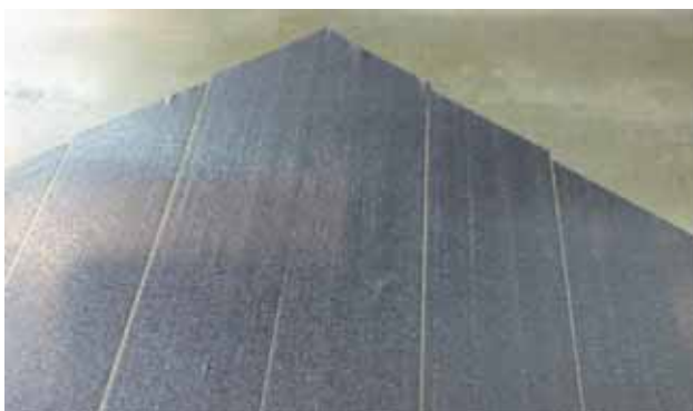
Picture 4. Gaps and overlaps
