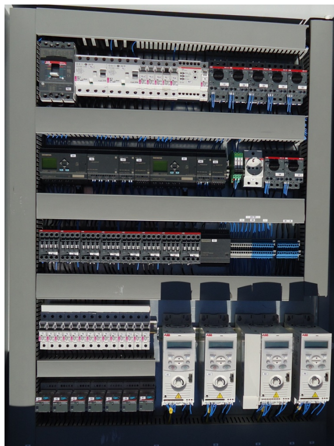
Figure 5: The electrical cabinet for automation of the fountain.
