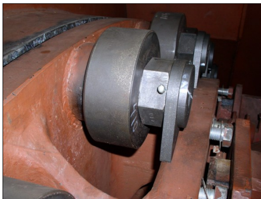
Figure 6. Pressure accumulator mounted on turbogenerator n.1 in TPP Bitola
