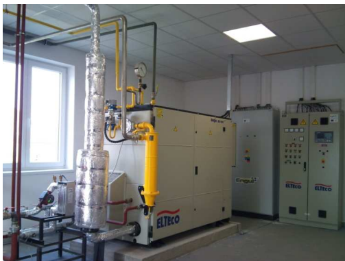
Figure 1. Apparatus of the National Centre - Cogeneration unit
