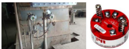
Figure 3: Pressure, flow, temperature transmitters used in the project
