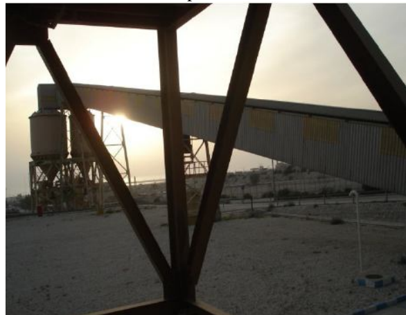
Figure 5: phase 1 conveyer to silo
