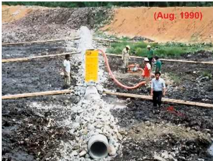
102. 9 - (Ampang Jajar , ) Figure 102. Measure 9 - Leachate collecting and venting pipe (Ampang Jajar Landfill, Malaysia)
