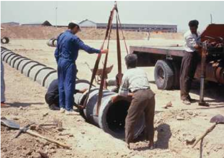
45. (Kahrizak , - ) Figure 45. Suitable placement example for ensuring perforation areas stay open (Kahrizak Landfill, Tehran-Iran)
