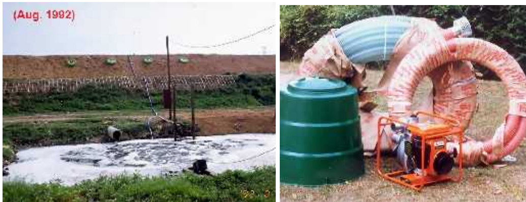
103. 10 - (Ampang Jajar , ) Figure 103. Measure 10 - Leachate collecting and venting pipe (Ampang Jajar Landfill, Malaysia)
