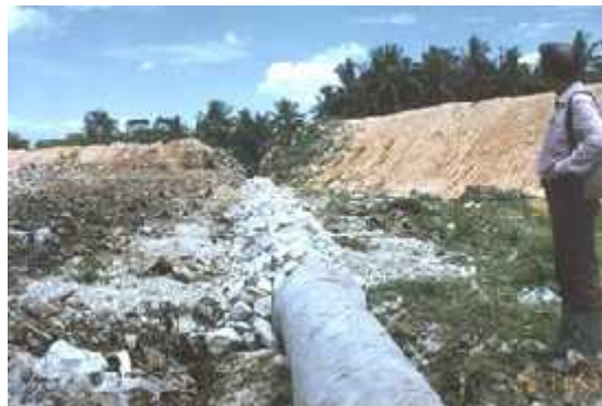
Figure 10. Sprinkle with stones between wooden stakes for stability from sinking (Ampang Jajar Landfill, Malaysia)
