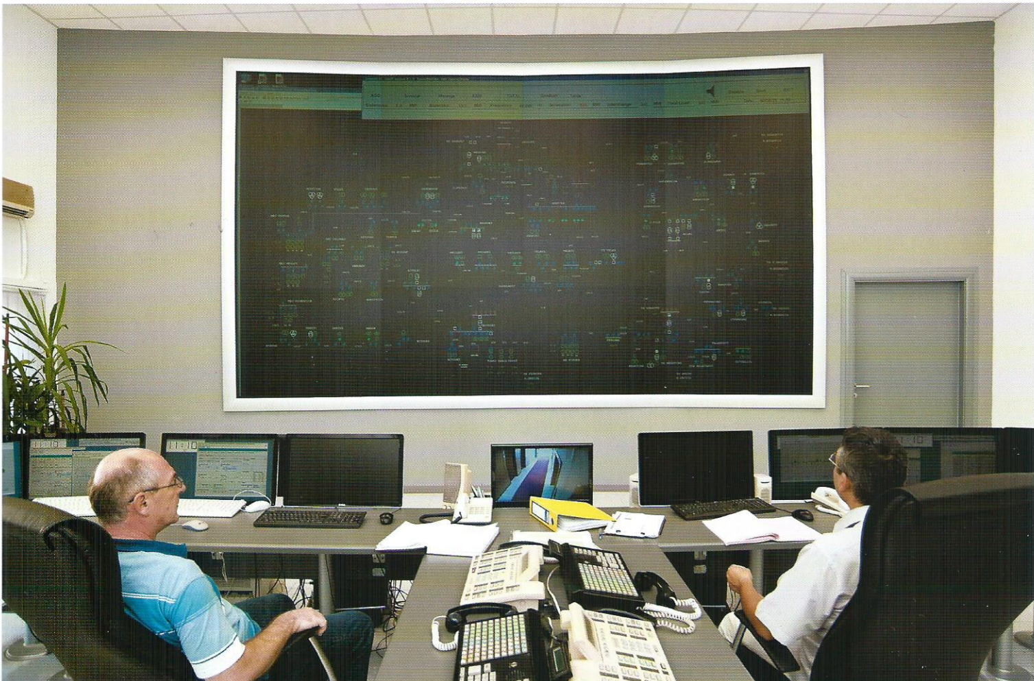
The MEPSO dispatching centre
